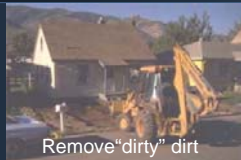
Remove "dirty" dirt
